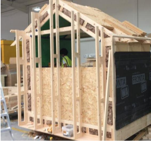
Production of the Passive House ice box: The design has been determined by a student competition. © Glasgow Ice Box Challenge
