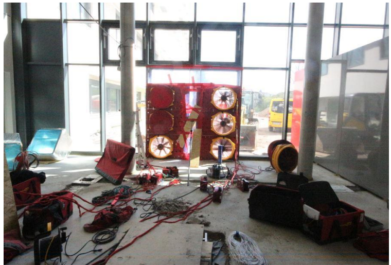
The pressure test inside the Passive House hospital in Frankfurt, Germany: more than 2000 rooms on eight storeys had to be inspected in advance, including making sure that more than 1000 windows were shut. © Passive House Institute
