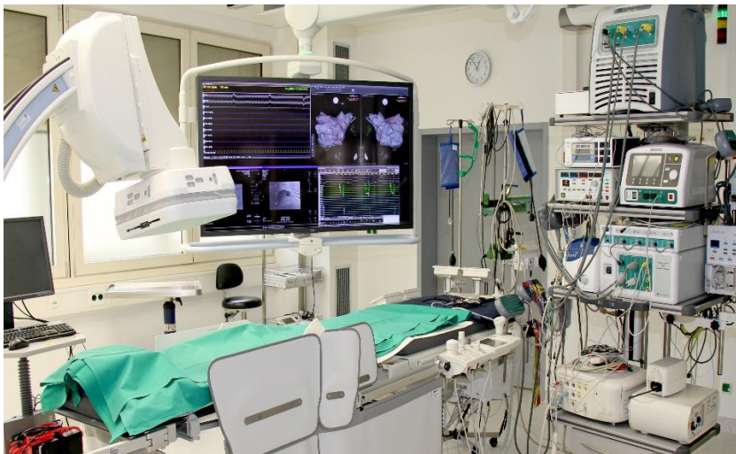
To determine the total energy demand for a clinic, all building facilities should be considered, including technical devices.
