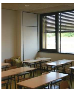
Ventilation units are inconspicuous in the rooms (white door).
