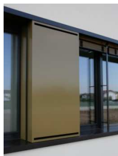
The air intakes and outlets seen from the outside.
