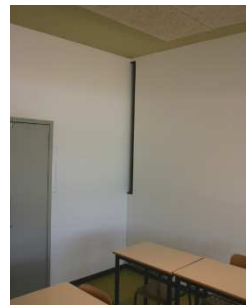
Air outlet situated in the corner of one of the new classrooms.
