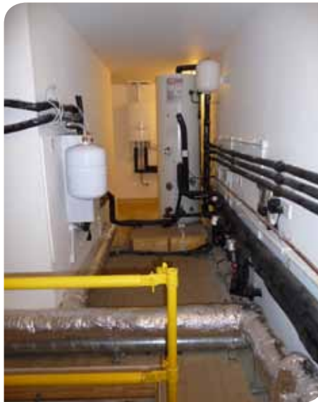
Building services, Racecourse, Gentoo Homes
