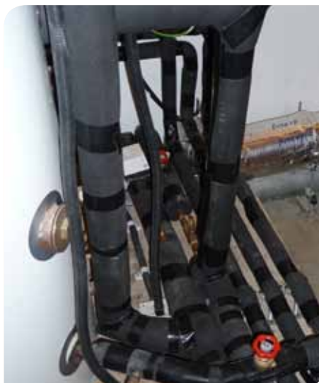
Insulated DHW pipes
