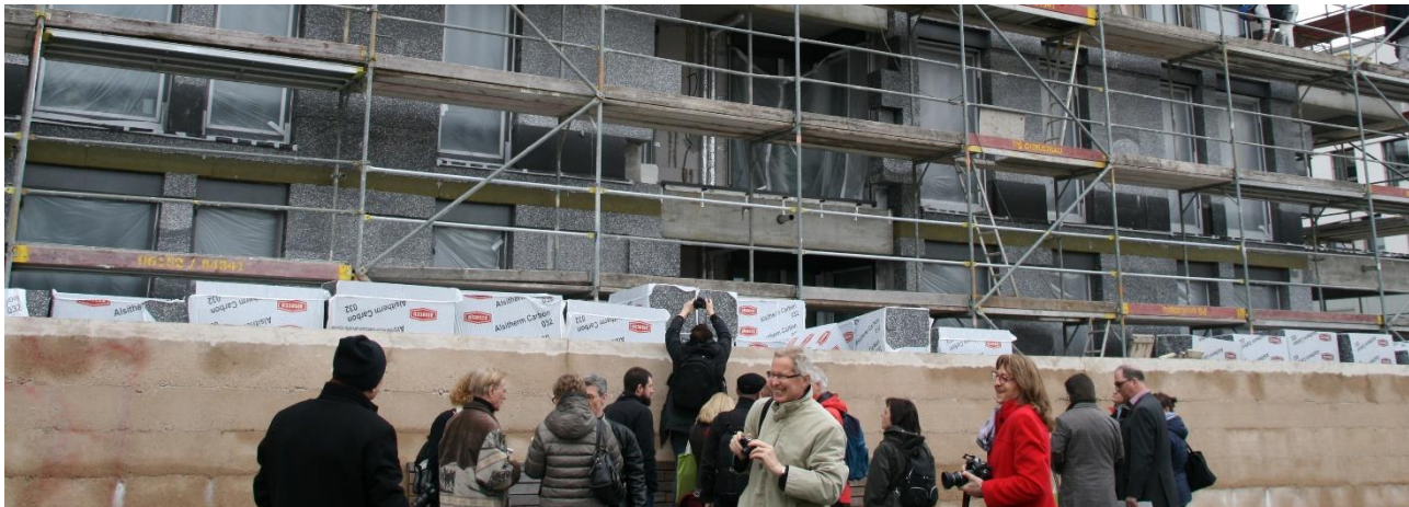
There was great interest in the information event on the energy monitoring of Heidelberg's Bahnstadt. The Passive House city district consumes two thirds less energy than typical complexes.. Photo: Passive House Institute
