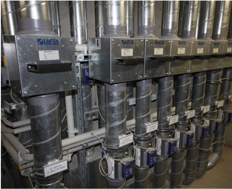
Despite the ventilation system in each apartment, the electricity consumption in Bahnstadt is well below the average. Photo: Passive House Institute
